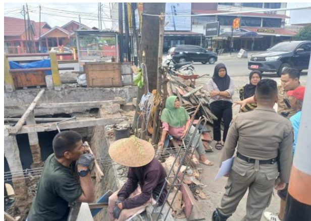
Figure 3. Enforcement of an Illegal Structure on Public Infrastructure
