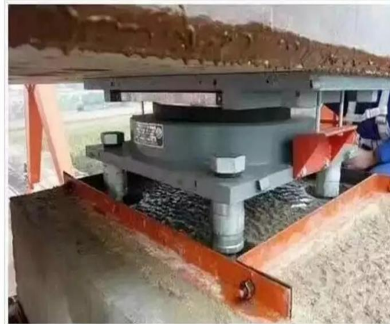
Figure 3. Installed Seismic Bearings
