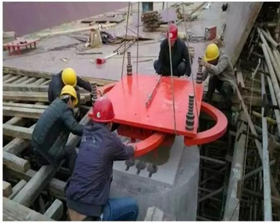
Figure 2. Installation of Seismic Bearings to Reduce the Impact of Earthquakes on Building Structures
