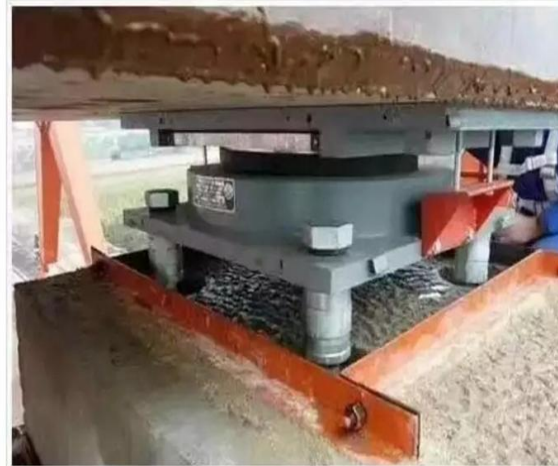
Figure 3. Installed Seismic Bearings
