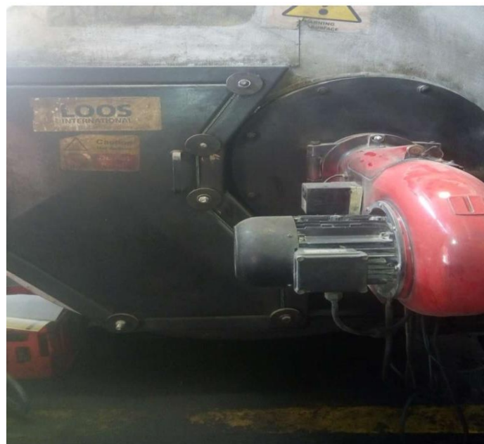
Plate 4.0: front view of the boiler
