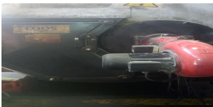
Plate 4.0: front view of the boiler
