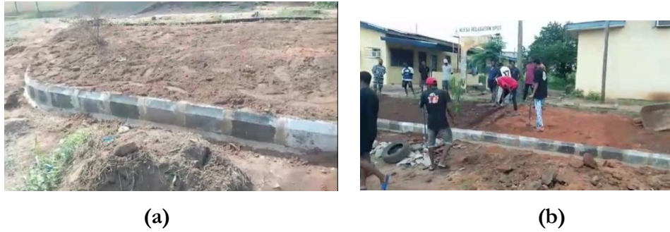
Figure 5: (a) Cut and fill process; (b) Sand filling and levelling of CVE Area
